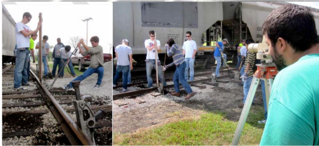
Fig. 3: UIUC RailTEC performing field work at Monticello Railway Museum in Monticello, Illinois (Lautala et al. , 2011)
